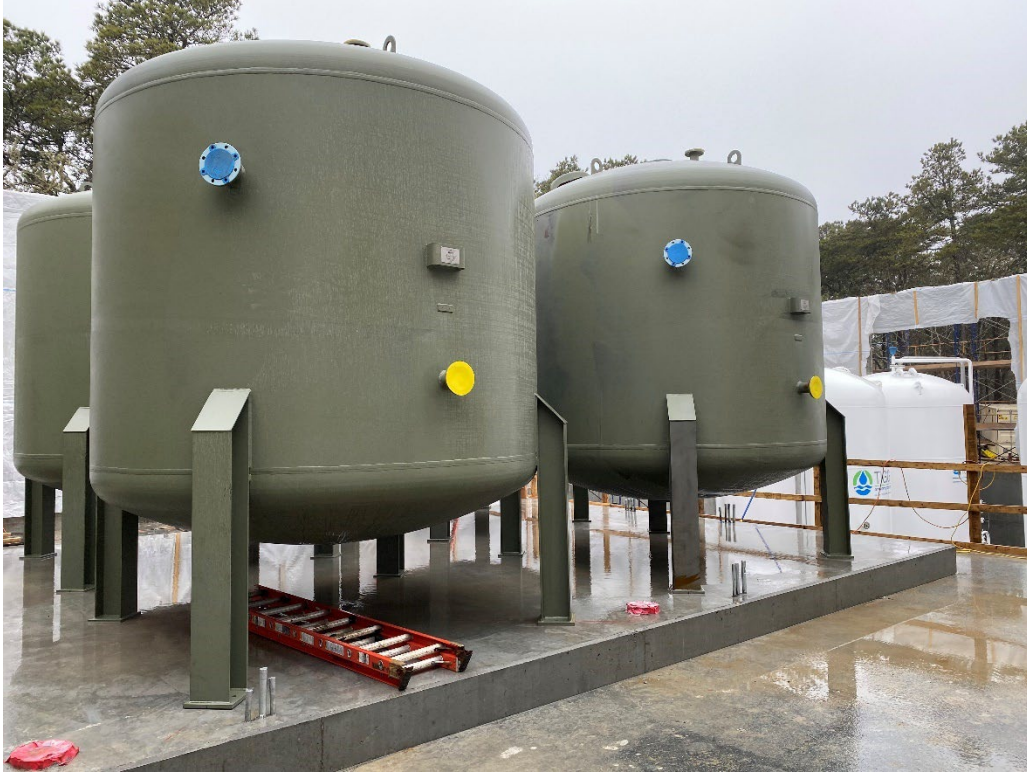
Wells 5 & 8 Treatment Plant – Green Sand Filters
