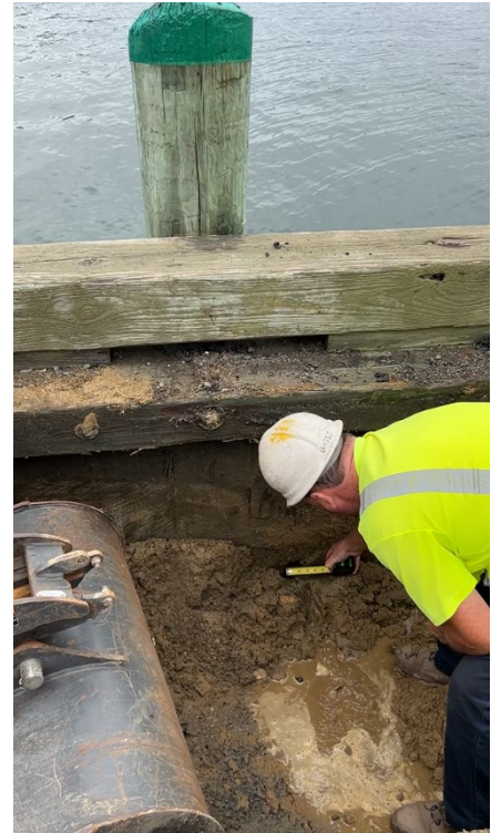
Above: A leak in the Ryder’s Cove bulkhead was identified in Fall 2025, prompting a temporary repair.
