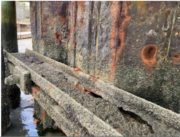
Above: Photograph from the bulkhead inspection showing widespread corrosion of bulkhead.
